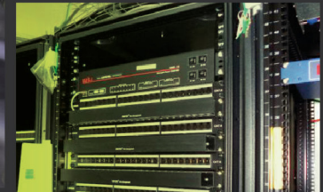
IT equipment installation BBC WS Dar Es salaam Tanzania
